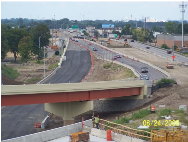
Looking north at the southbound I-75 lanes as well as the new exit ramp to northbound SR 4/Webster Street.
